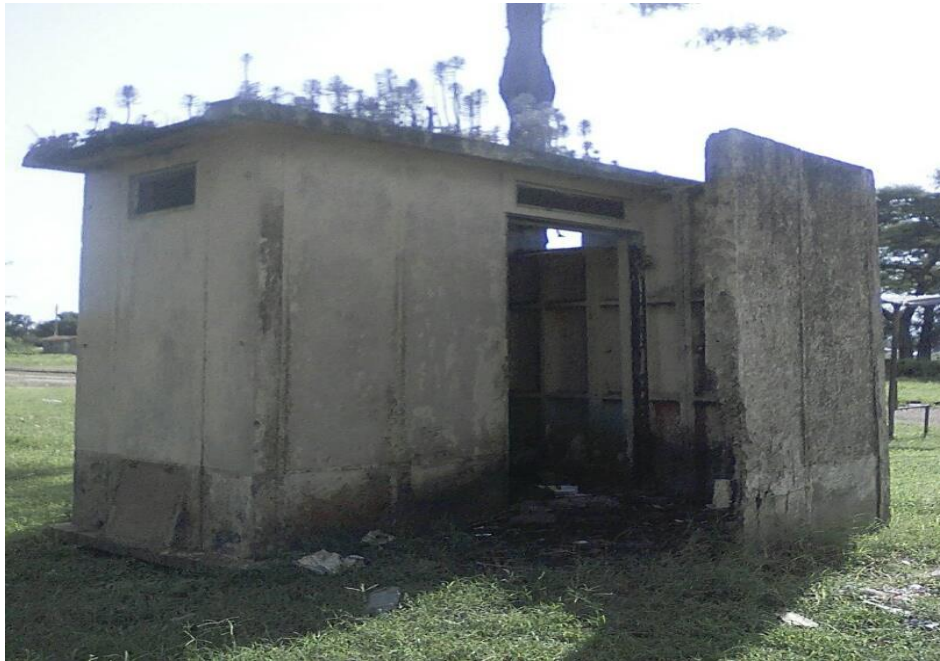
Figure 12: A dilapidated pit latrine in Muhoroni town
