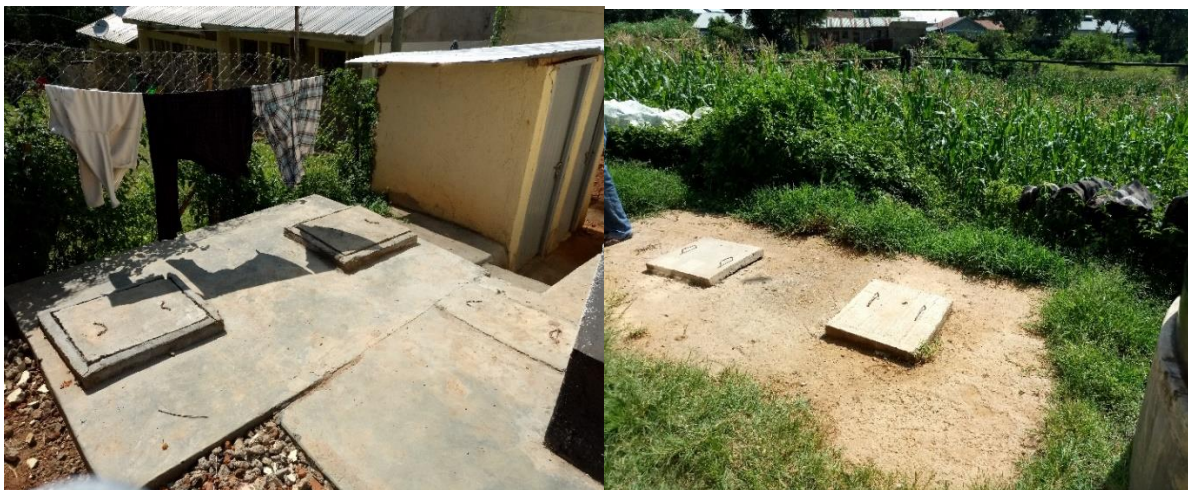
Figure 14: Pour flush to a septic tank at Sondu and Septic tank at Maseno
