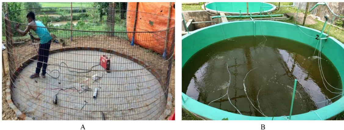
Fig. 3. BFT tank construction process using wire mesh (A) and concrete material (B). Picture courtesy of Mr. Debtanu Barman (CEO Aqua-Doctor Solutions Co. Ltd, India).
